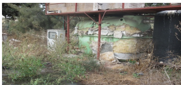
Photo (4): the desalination machine in Al- Aroub
