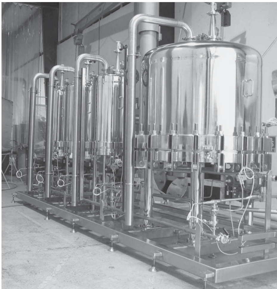
Figure 16.7 Industrial-scale depth filtration system for cell harvest and clarification. (Reproduced with permission from Cuno Incorporated).
