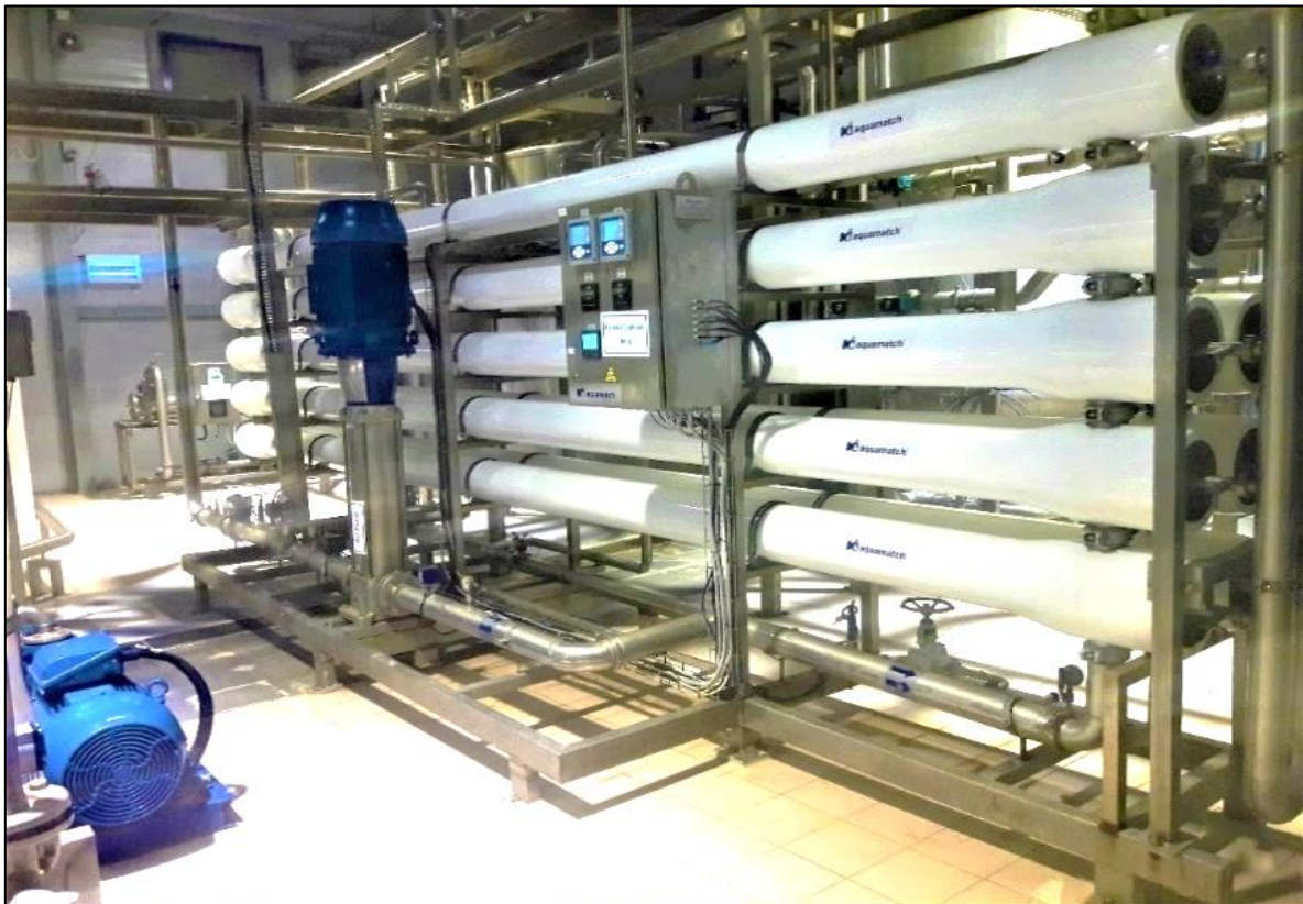
Figure (2.8): Reverse Osmosis main unit in Pepsi Plant in Jericho City.
