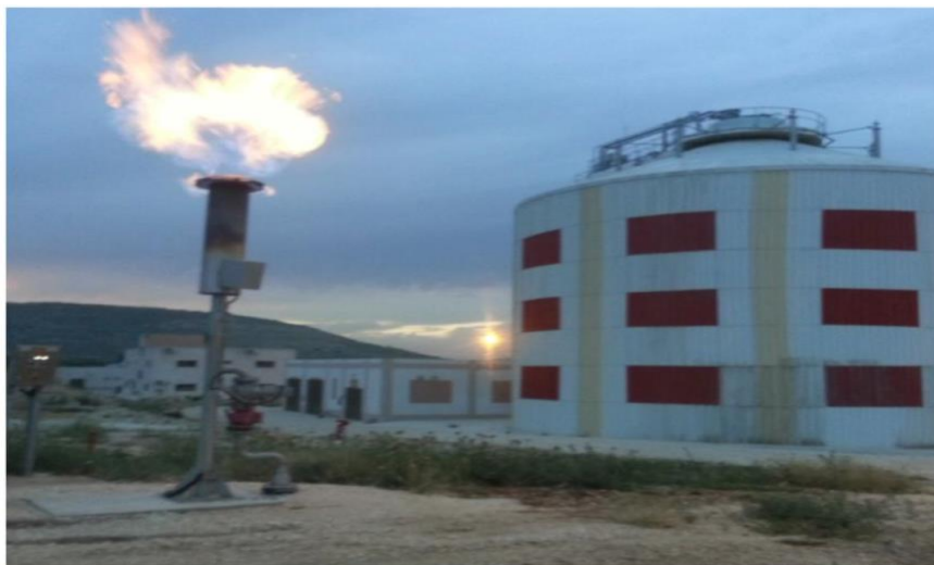
Figure 12, Digester tank in Nablus West WWTP with the gas flare (West & Yousef Abu Jaffal, 2022)
